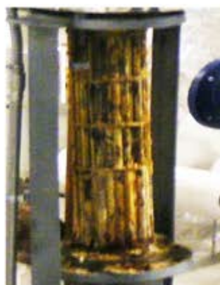
Limescale buildup on a heat exchanger before Flow-Tech
