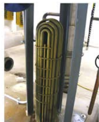
Flow-Tech removed existing scale, and prevented new scale, restoring performance
