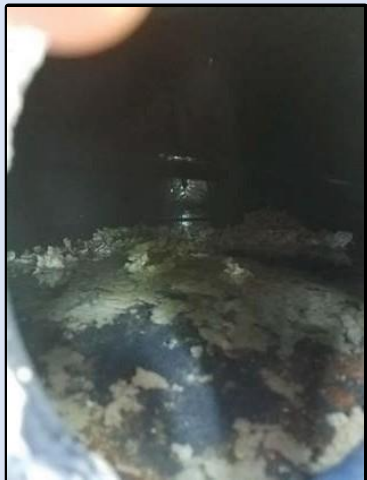
After four months, the heater tubes remained clean and kept their energy star ratings.
